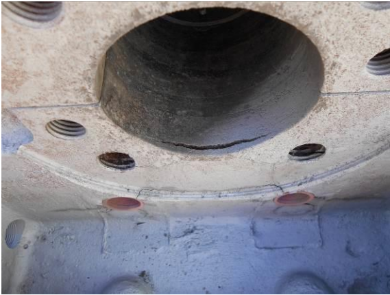
Figure 17: Pump Water Jacket Cracked
