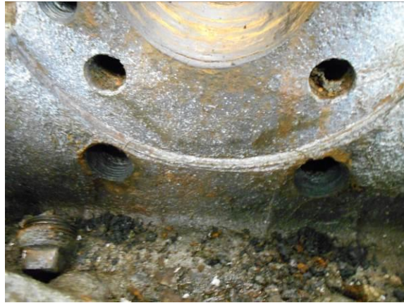
Figure 18: Debris from Cracks Cleaned Out
