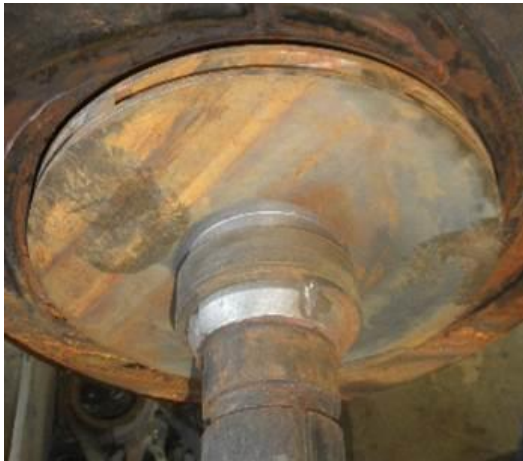
Figure 3: Original Impeller Condition on Shaft
