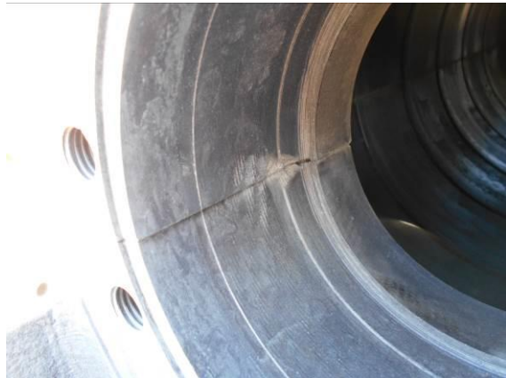
Figure 19: Wear out on Thrust End Left Side
