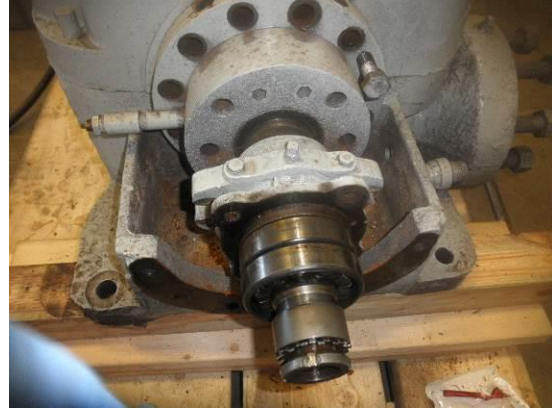
Figure 46: Original Thrust End Bearing
