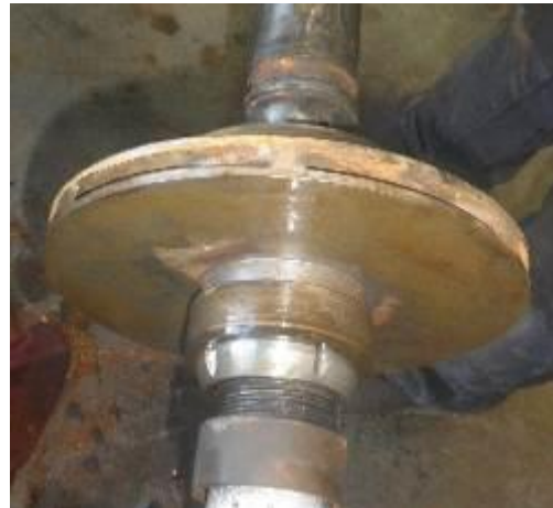
Figure 4: Original Impeller Condition on Shaft
